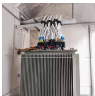
Transformer station underground parking garage 4 Trafos à 1600 kVA
